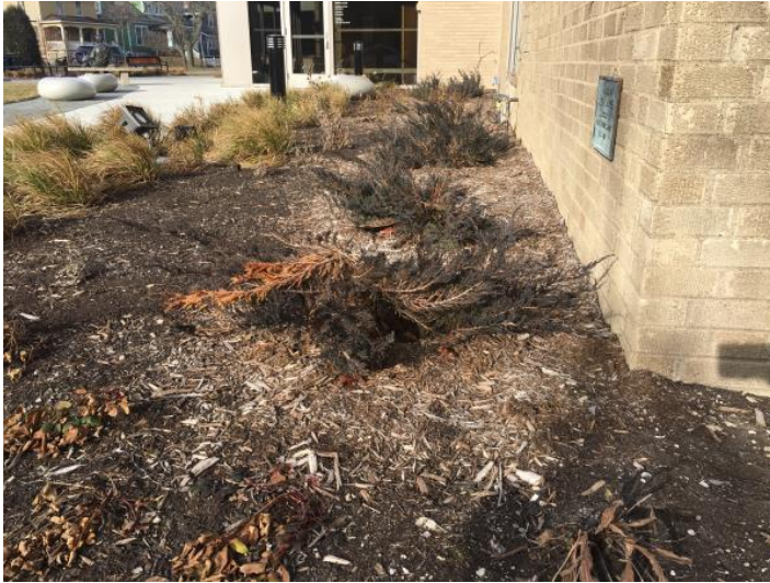
Top: Landscaping along west wall above brick ledge and area well Bottom: Landscaping above brick ledge south side of building
