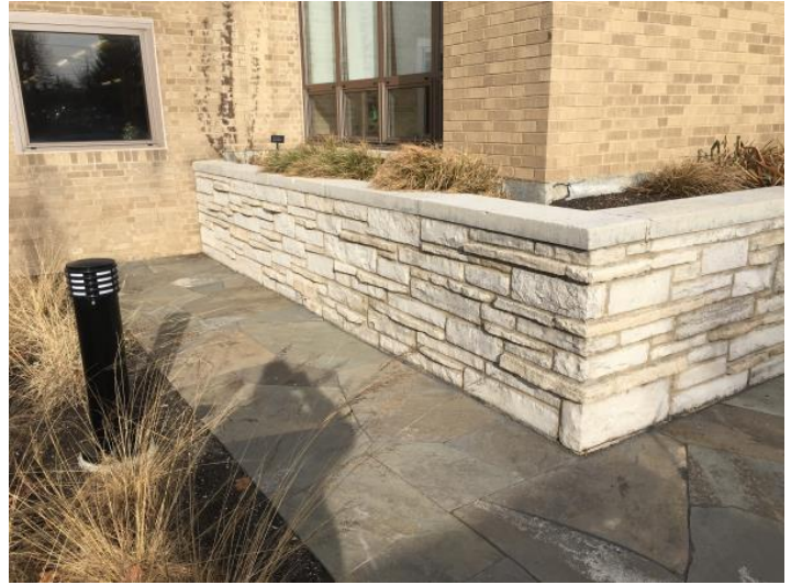
Top: Elevated planter wall extending past raised foundation wall and flashing in disrepair Bottom: Sidewalk at door east of elevated planter above brick ledge
