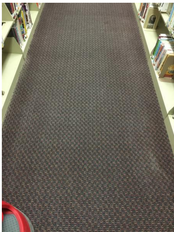
Top: Stained carpet in basement Bottom: Water damage along south foundation wall
